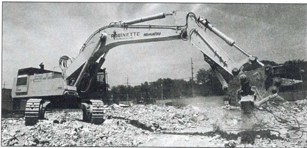
Robinette Demolition's NYE digital concrete pulverizer Series 7 works on a Komatsu PC-650.
